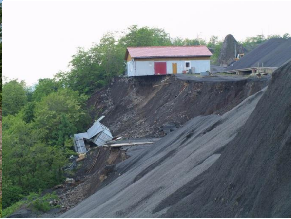
Fig. 3: Damages in the Dobkovičky quarry.
