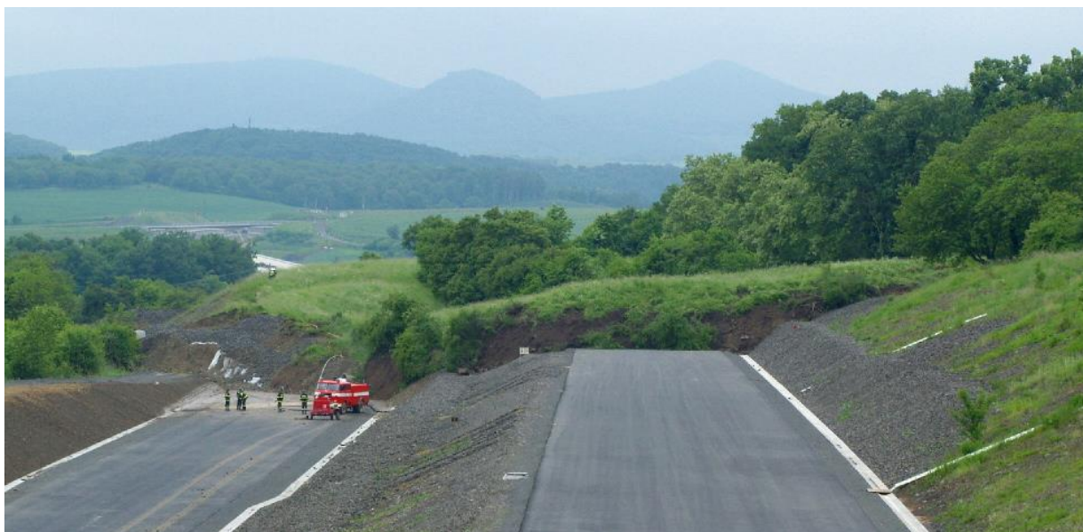
Fig. 1: Damaged motorway D8 which was under construction at the time of landslide.
