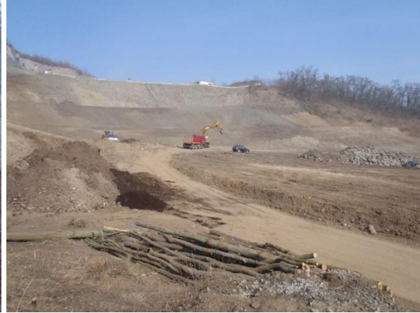
Fig. 7: Final form of landslide in the upper part.
